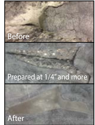
Surfacing in a food plant with KIRC9000. 15min hardening. 1h for lifts to roll over..
